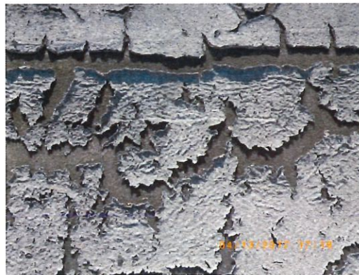
Photo 2: BUR systems of similar age and construction that were coated experienced visible damage and separation of the stone aggregate (Photo by Ralph Moon)
