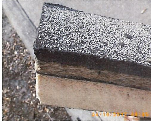
Photo 1: Cross section and appearance of a BUR that was not coated in the energy savings program (Photo by Ralph Moon).
